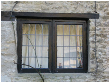
The contrast between traditional and replacement finishes on windows in the village
